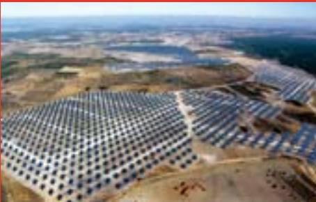
Europe's largest solar electricity farm, in Amaraleja (in the municipality of Moura), Portugal.
