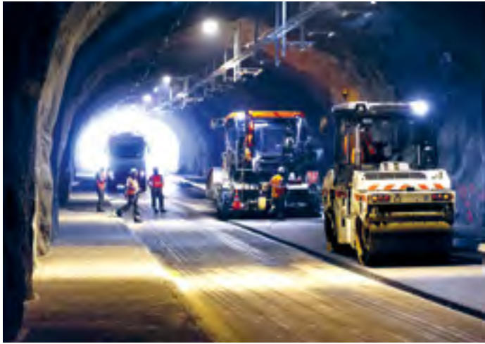
Le Freney-d’Oisans — The Chambon tunnel, which had been closed since 2015 due to a landslide, reopened to traffic in December 2017.
