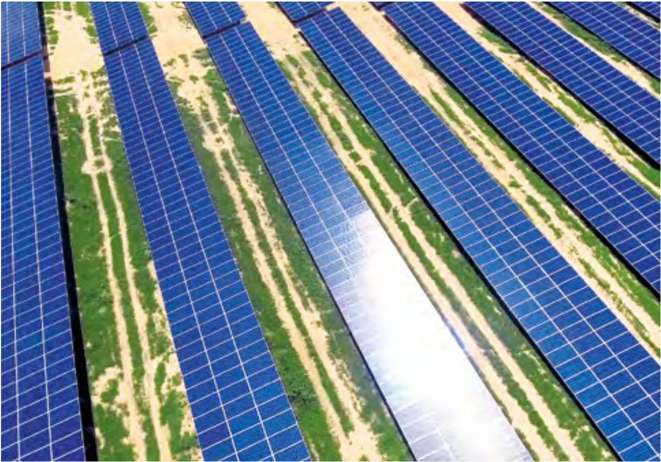
Ten Merina (Senegal) — Photovoltaic power plant.
