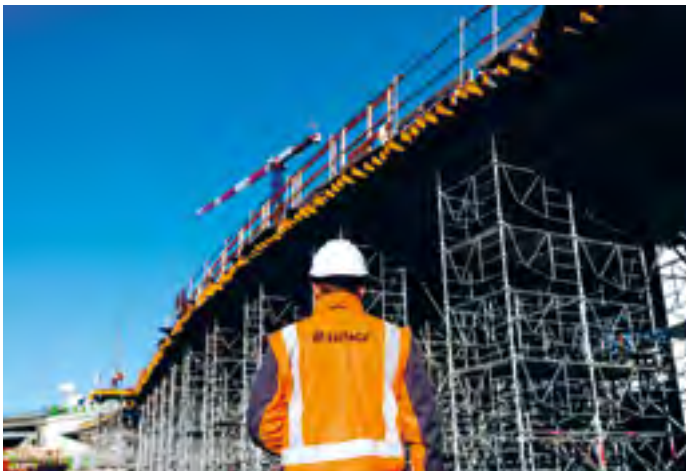
Paris — Eiffage Génie Civil is carrying out work to restructure the Quai d'Ivry interchange on the city's inner ring road, located within the Paris Rive Gauche development zone.
