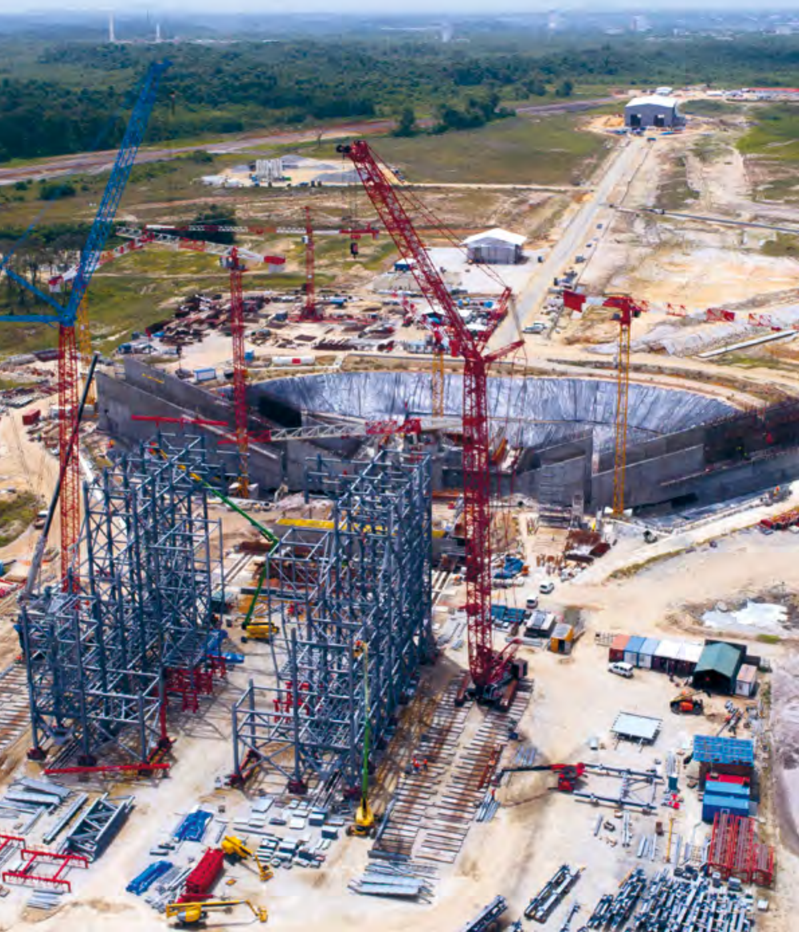
Kourou (French Guiana) — Eiffage is building the Ariane 6 launch complex, via an integrated offering
